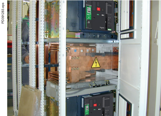
Source changeover system in the same cubicle.
