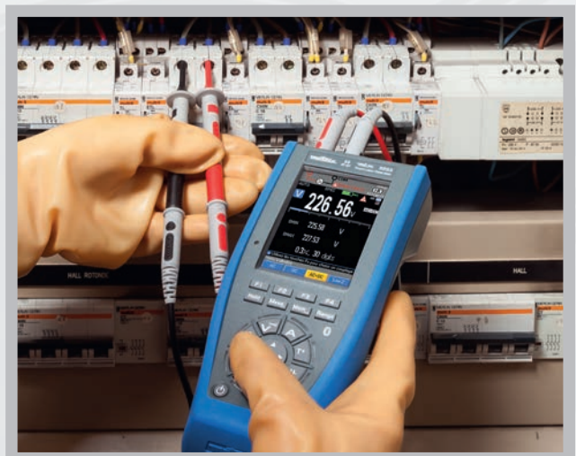
Measurements on electrical cabinets
