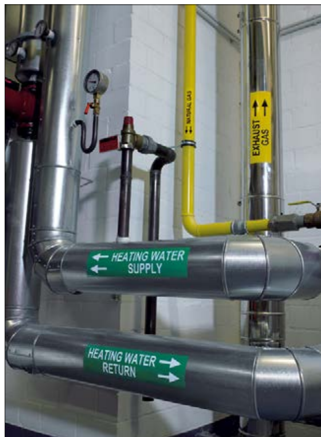
Large and highly visible pipe marking.
