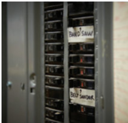
Label electrical components: 3M™ Masking Tapes ( pgs 57-60 )
