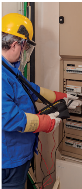
Control of an electrical cabinet
