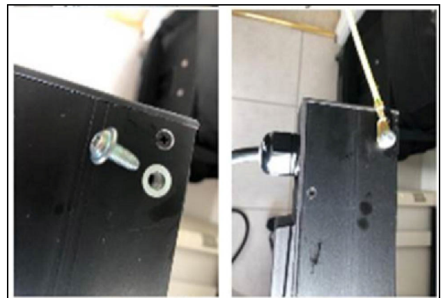
Fig. 15: Housing earthing point of the PDU
