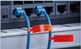
Communications and power
